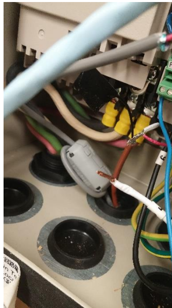
Figure 6.8 A partially disentangled wire nut connection. The white wire to the brown cable must still be disconnected
