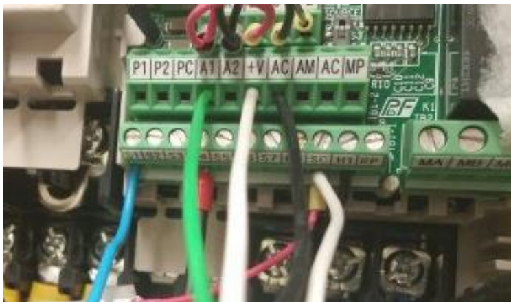
Figure 6.6 A rewired VFD. The two white wires are not connected to each other
