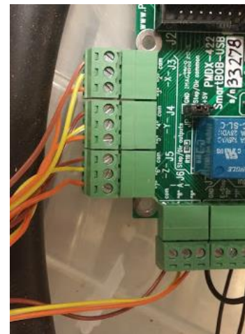
Figure 4.10 Yellow wires carry step pulses, orange carry direction, and brown set the reference voltage
