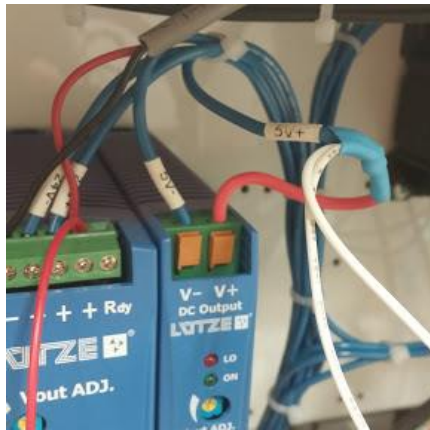
Figure 4.9 Wires leading from the power supply
